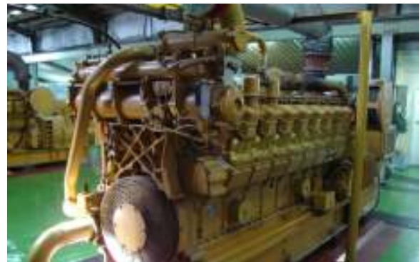
Fig. 11: 1 MW diesel engine.
